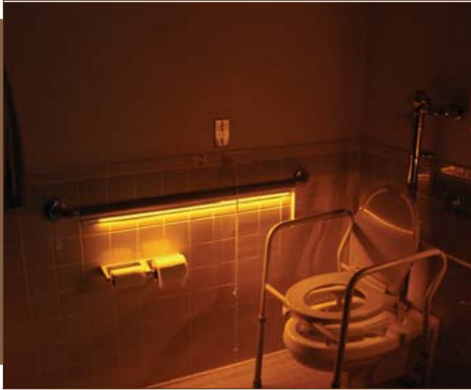
(Figure 8) Amber LEDs light below grab bars to provide sufficient light for navigating at night, but not too much to startle you from sleep.
